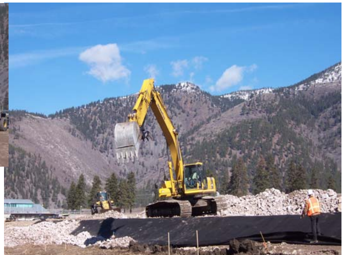
Hauling and Placement of Rip Rap on the Clark Fork River Flood Berm
