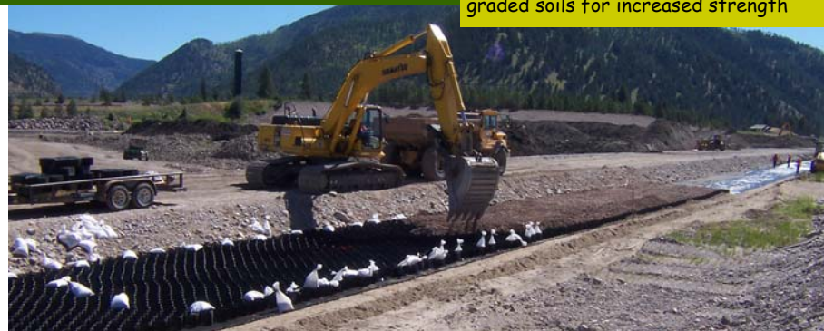
Construction of the on-site rail spur using a geo-grid filled with specially-graded soils for increased strength
