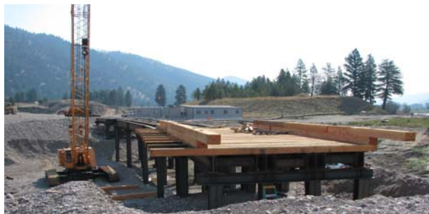
Construction of the rail bridge on site. Installation of decking. This will be the only way to cross the bypass channel and is designed to carry rail cars loaded with sediments, vehicles, and foot traffic.
