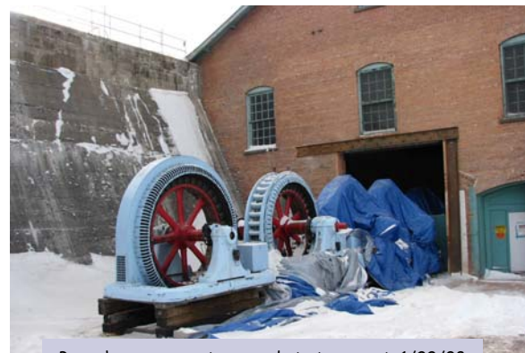
Powerhouse generators ready to transport, 1/22/08
