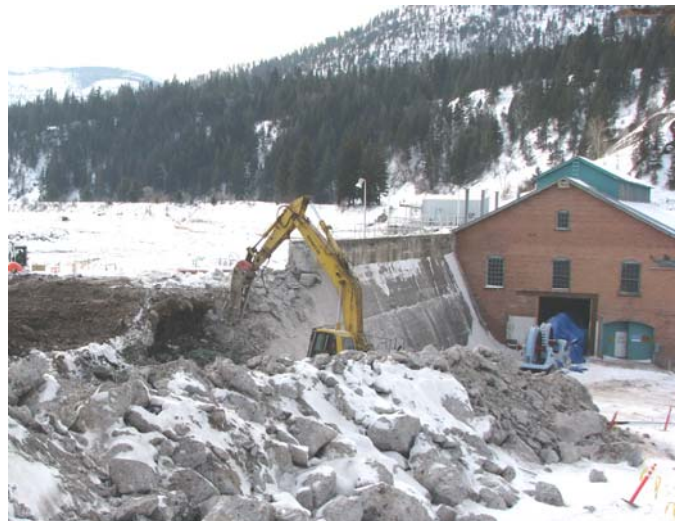
Removal of the right (north) abutment wall of the Milltown Dam Structure, 1/22/08.
