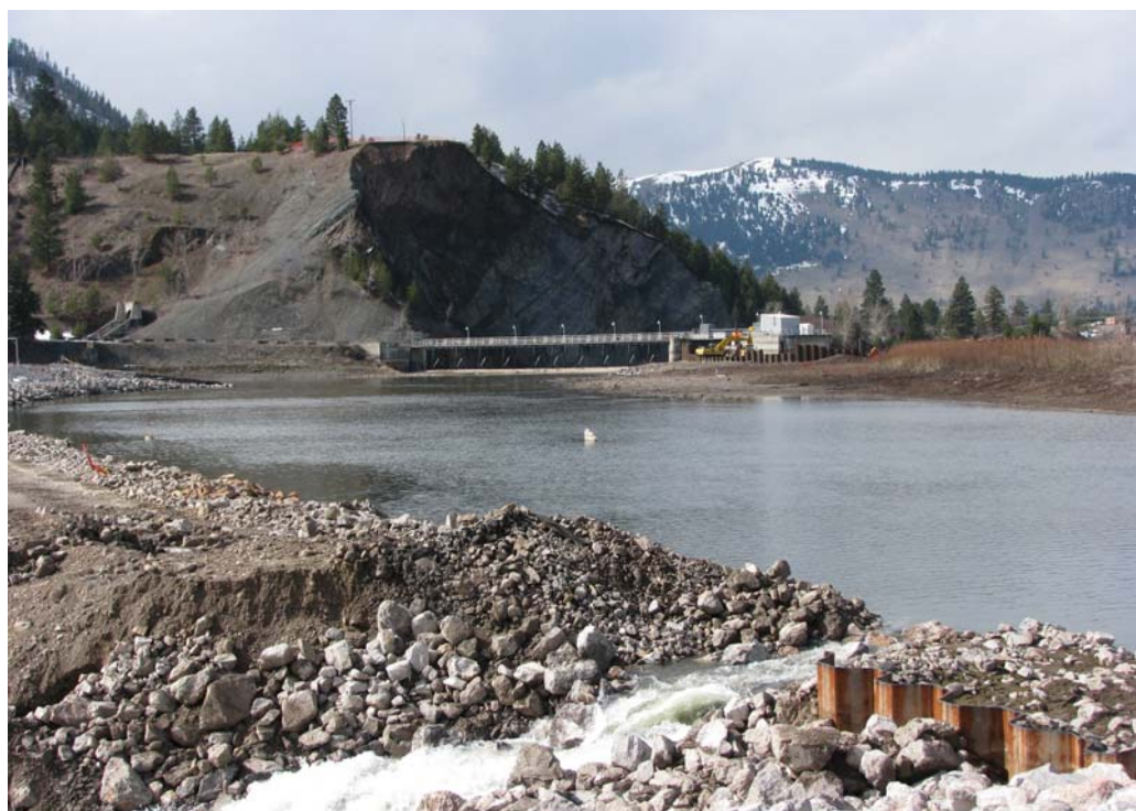
The outlet of the bypass Channel was opened yesterday, March 18, 2008, allowing water from the Blackfoot River to flow into the channel. It took 14 hours and approximately 44 million gallons of water and now the water level in the bypass channel is filled.
