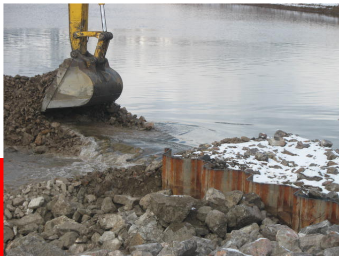
The photo to the left shows the excavator removing the final barrier to open the bypass channel outlet to the Blackfoot River. (March 18, 2008)
