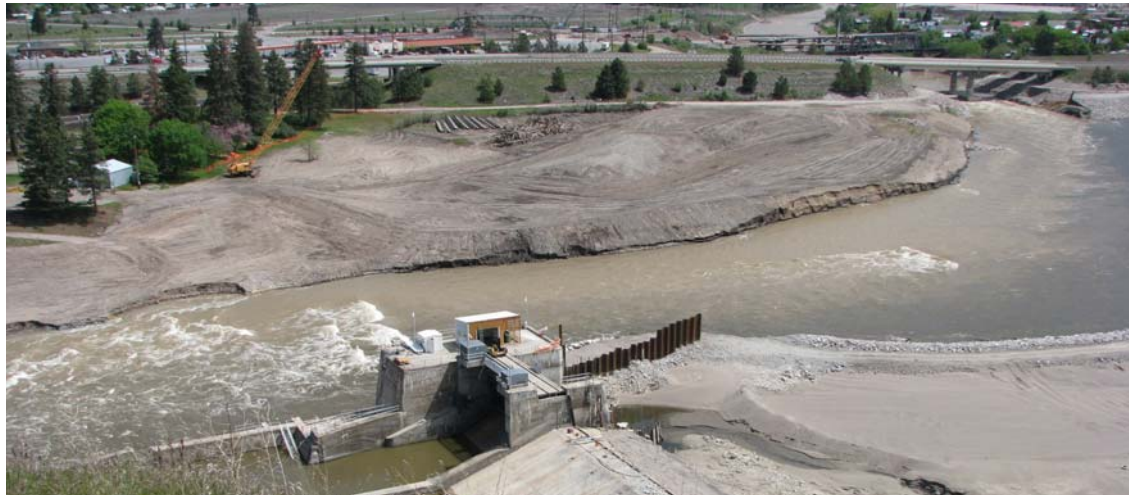
View of the confluence of the Clark Fork and Blackfoot Rivers. Workers are beginning to remove items located on top of the Divider Block in preparation for removal of the remainder of the Milltown Dam. Photo taken May 28, 2008.
