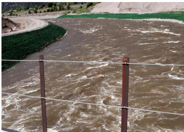
View of the flow in the Clark Fork River Bypass Channel. Photo taken 5/26/09 by Kris Cook of Envirocon, from the on-site rail road bridge.
