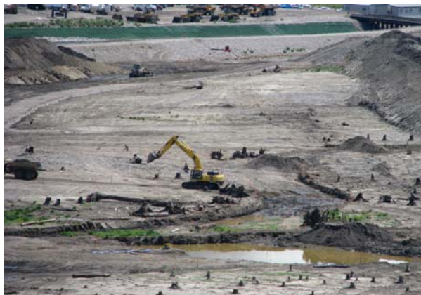
Digging a new river channel in the former reservoir area. Note stumps from original floodplain.
