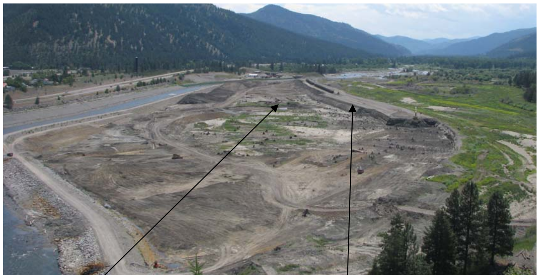
View of Project Area from Milltown Overlook, 7/7/09. The new Clark Fork River channel and floodplain are beginning to take shape. Notice the shortened rail line and excavation from underneath and around the former rail line footprint.
