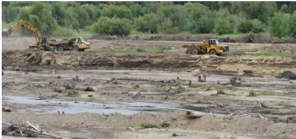
Hauling material from upstream to on-site repositories as part of site restoration, 7/14/2010.
