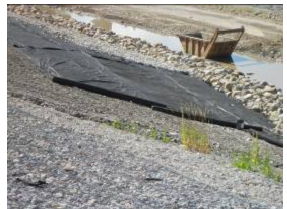
Placement of geo-textile on the slope along I-90. This work is part of the removal and regrade of the bypass channel. Placement of reno mattresses should be done in August; the regarding/restoration should be complete in September 2011.
