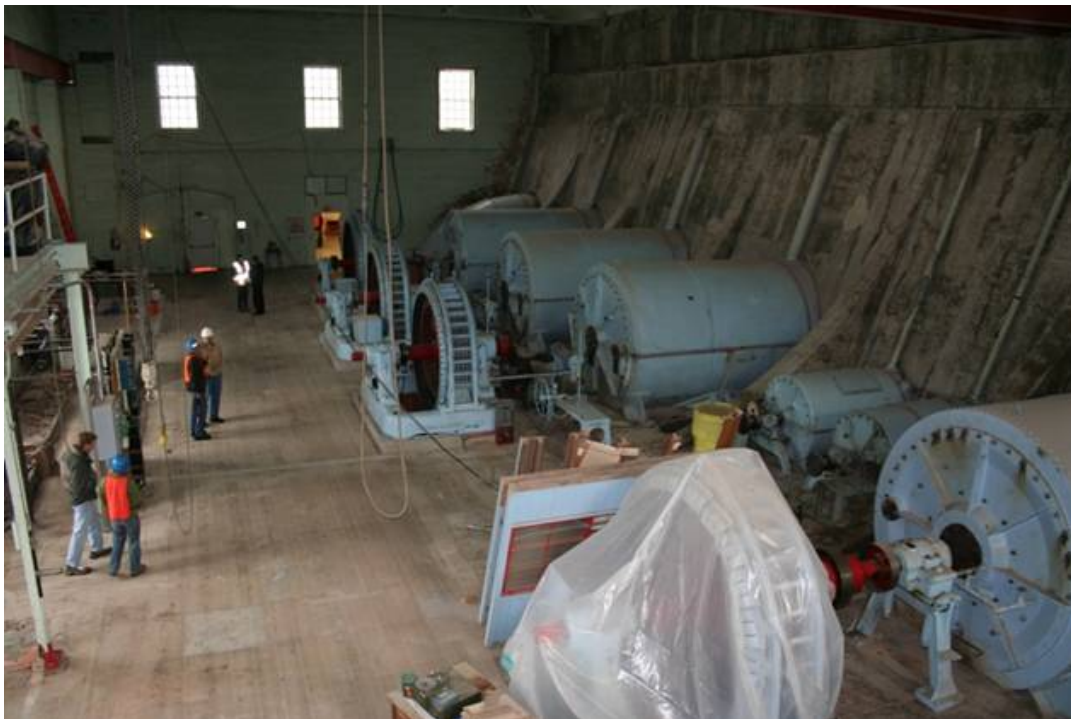
This photo of the powerhouse interior was taken in December, 2007. The lead based paint has been removed from the powerhouse floor and the headwall, at the right side of the photo.
