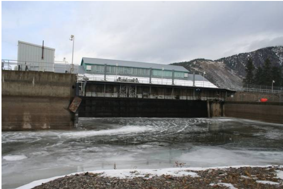
The photo above shows a view of the powerhouse forebay, looking downstream at the dam. This area will be the site of construction activity to prepare of the powerhouse removal, beginning this month.
