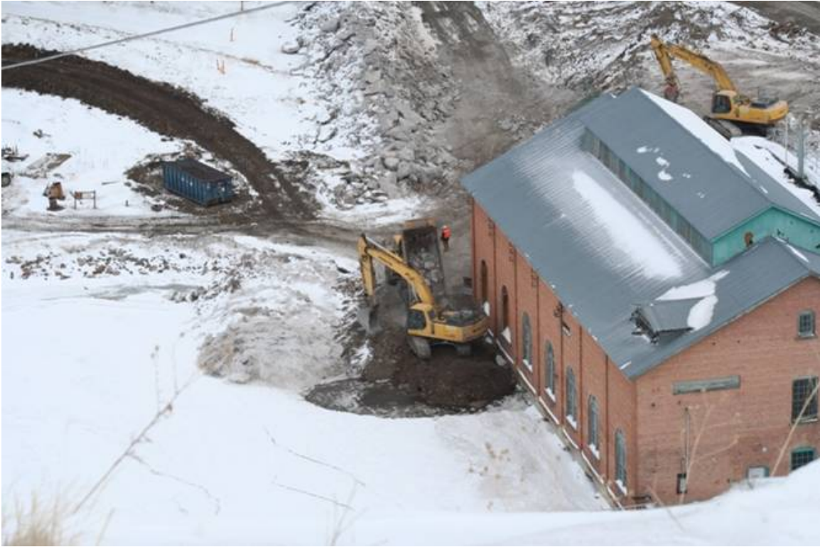
In the photo above, taken yesterday from the bluff overlooking the dam, an excavator is building a work pad downstream of the powerhouse that will be used during its demolition. The work pad will also keep water in the river below from flowing back into the excavation area.
