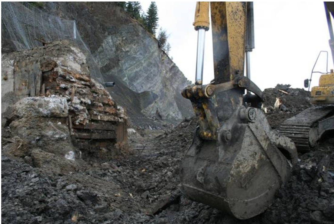
On October 7, 2008, the left abutment removal was nearing completion. Remnants of the original timber crib remained, stained by years of immersion in the reservoir by iron and manganese. Globes of concrete grout poured out of the old timber cribs, where it had been injected to stabilize the rock fill and spillway.
