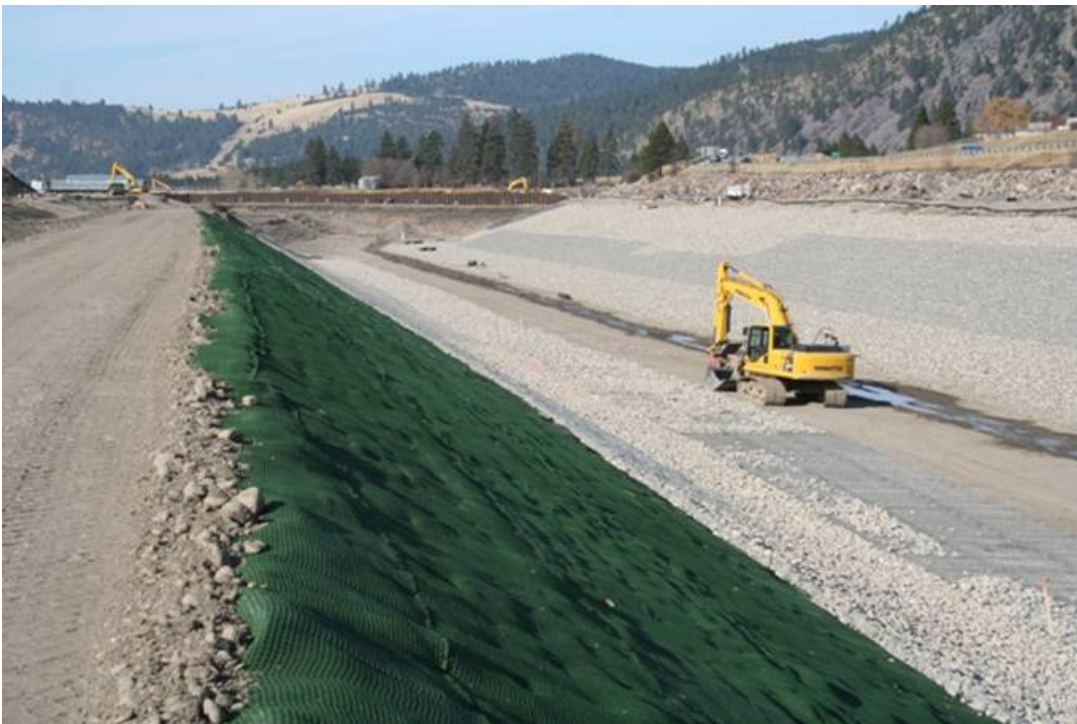
The bypass channel is being lined with rock filled wire baskets, called reno mattress, and green turf reinforcing fabric. The river may be diverted into the bypass channel next spring. The channel is sized to handle the 100 year flood after dam removal, and will remain in place for at least two years while the remaining contaminated sediments are removed.
