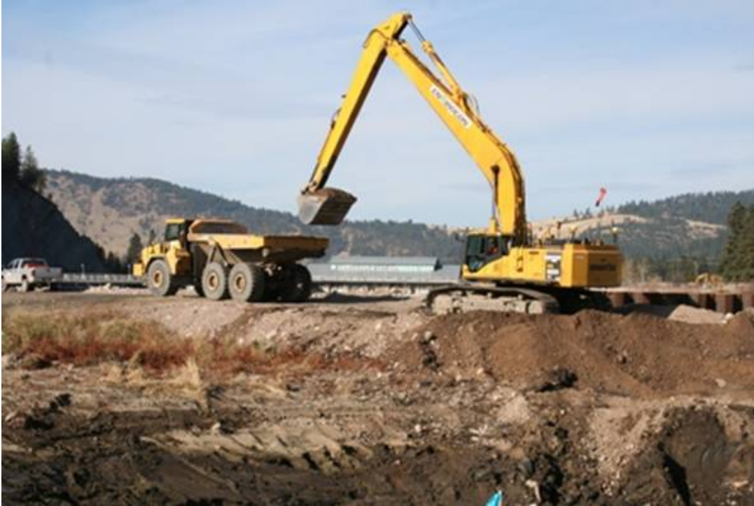
Excavation of the bypass channel is now nearly complete up to the outlet structure. The roof of the powerhouse is visible in the background.
