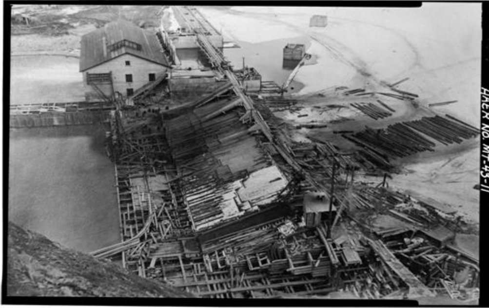
The photo above, courtesy of the National Archives, shows the Milltown dam under reconstruction in 1909. Note the construction methods of the time, using ten inch timbers crafted into cribs filled with rock. The spillway was completely reconstructed in 1909, shored up over the years and covered with concrete following flood and ice damage in 1986.
