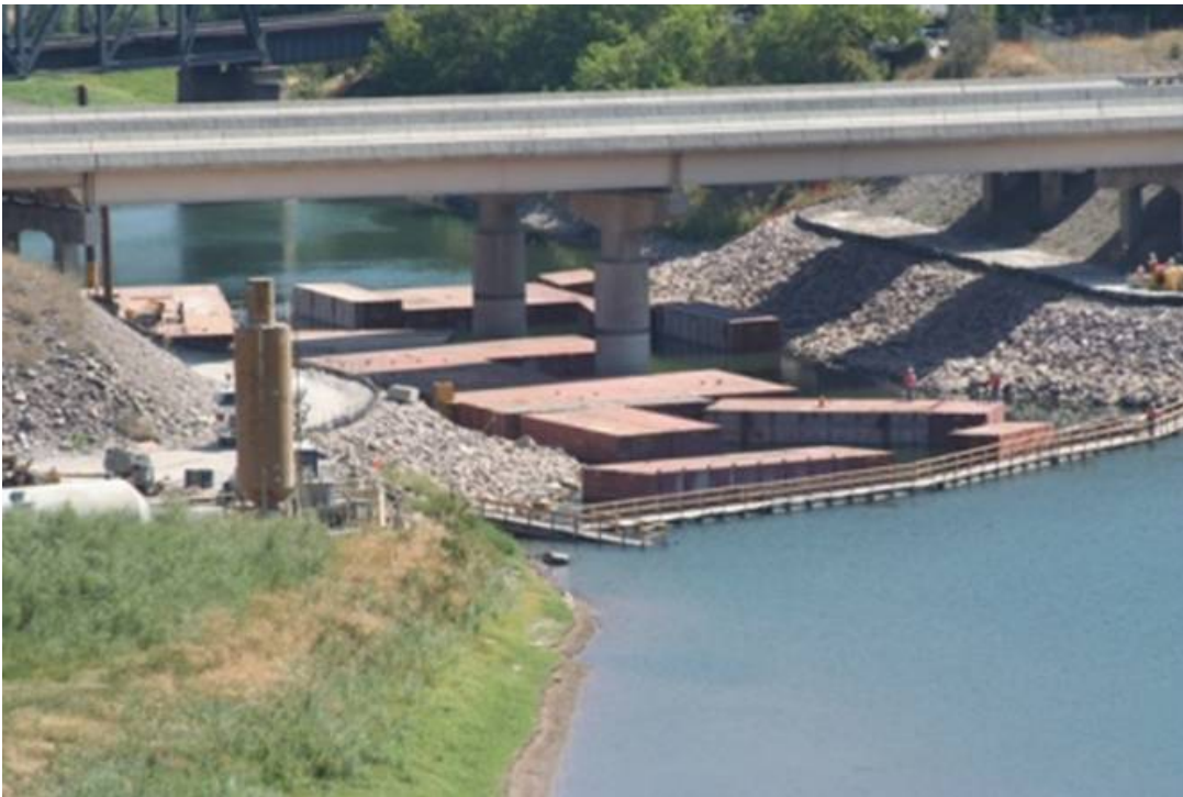
The U.S. Army Corps of Engineers has contracted with several construction companies to stabilize the Interstate highway bridges. Spaulding Construction, of Stevensville, is doing work on the slope stabilization and also completed the removal of timber cribs in the river behind the
