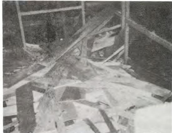
Picture of core waste accumulating at the No. 4 core station, prior to the modifications.
