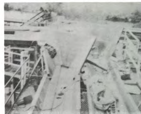
PLYWOOD MAINTENANCE Built a new 90 degree drop corner onto the Plywood Vat Infeed Chains
