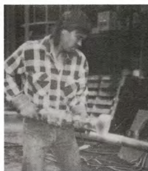
PAUL BARR of C.H. MURPHY COMPANY Boiler Repairs (tube replacement and fire wall repairs)
